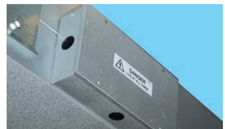
Built in control box.
